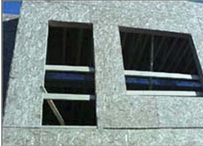
Figure 35 - Guardrails protecting window openings.
