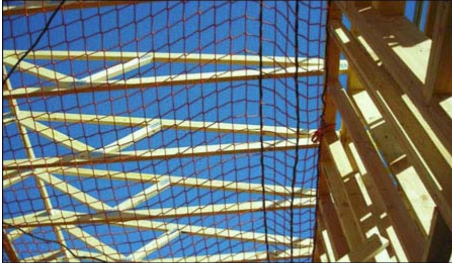
Figure 7 - An example of a safety net system.
