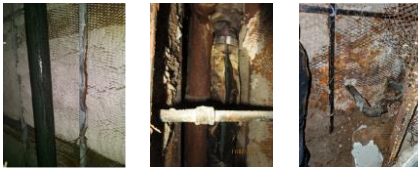
Missing insulation on cold water riser
