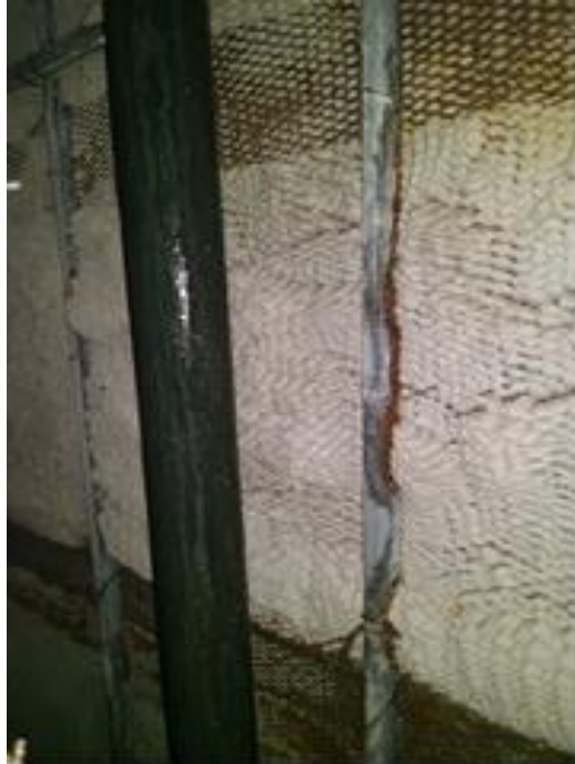
Missing insulation on cold water riser
