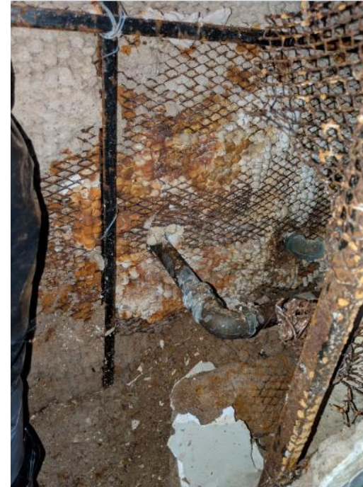
Missing insulation on cold water supply t
