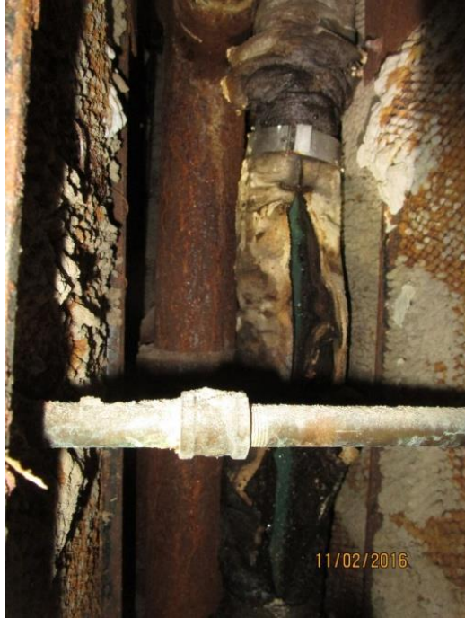
Damaged insulation on cold water riser
