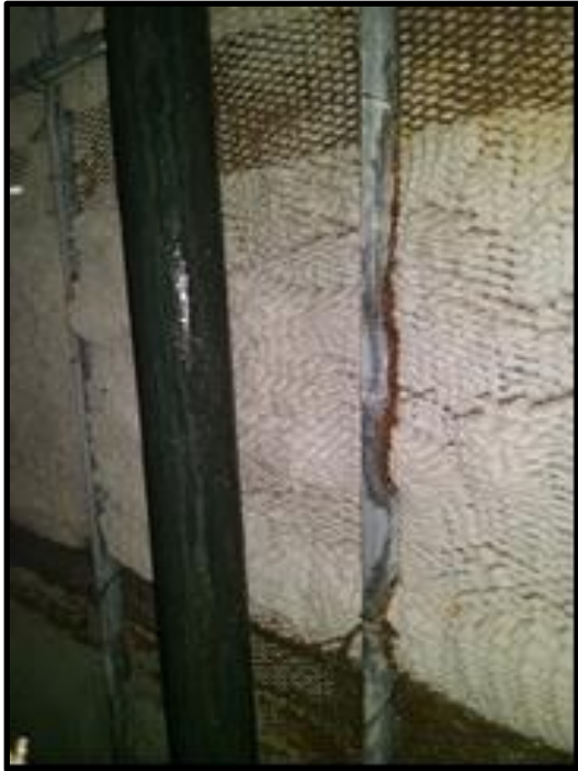
Missing insulation on cold water riser
