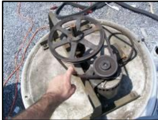
Loose or Broken Belts
