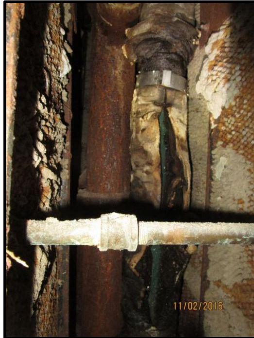
Damaged insulation on cold water riser
