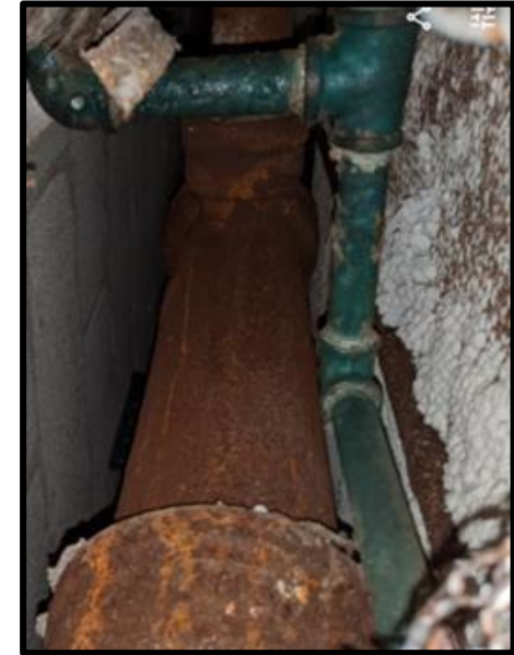
Example of condensation on the cold-water supply pipes.
