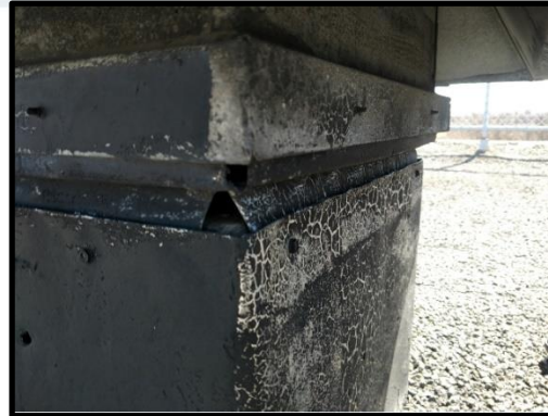
Improper Seating of Housing
