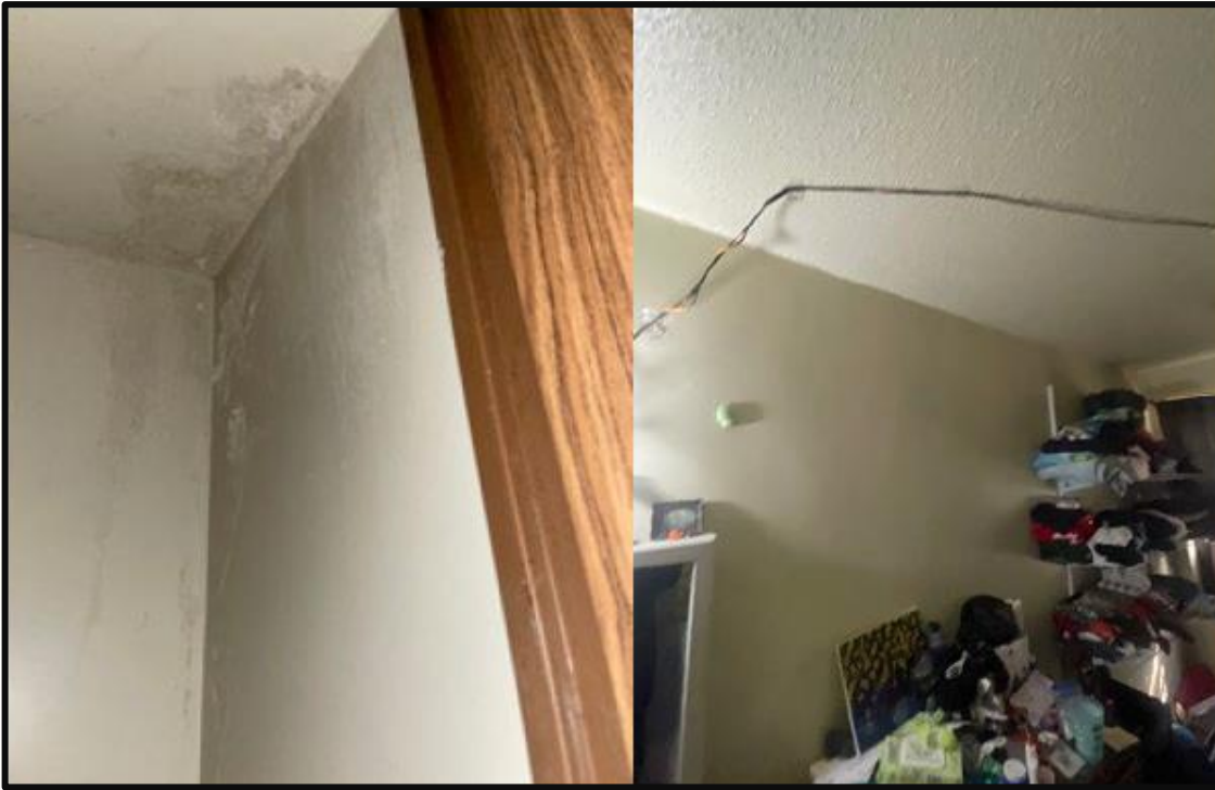
Water from an adjoining wall
