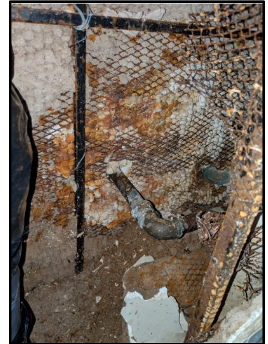
Missing insulation on cold water supply
