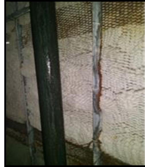
Example of condensation on the cold-water riser.
