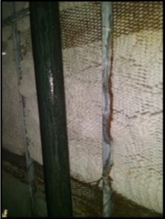
Missing insulation on cold water riser
