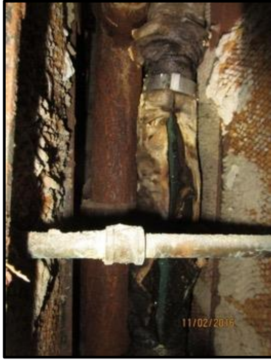
Damaged insulation on cold water riser
