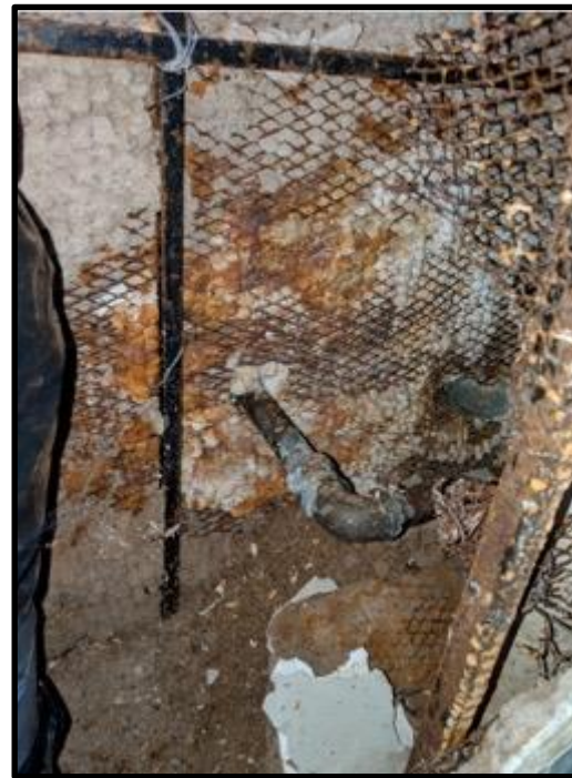
Missing insulation on cold water supply
