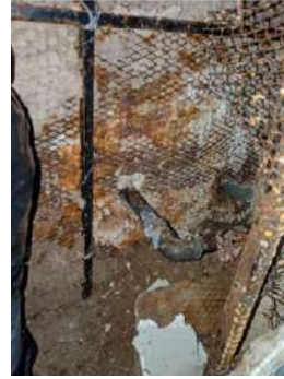
Missing insulation on cold water supply t
