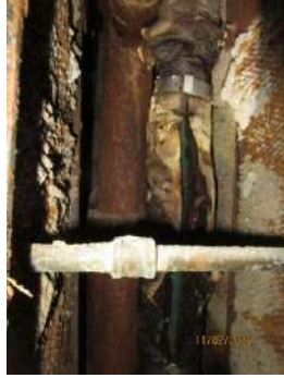
Damaged insulation on cold water riser
