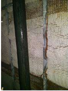
Missing insulation on cold water riser
