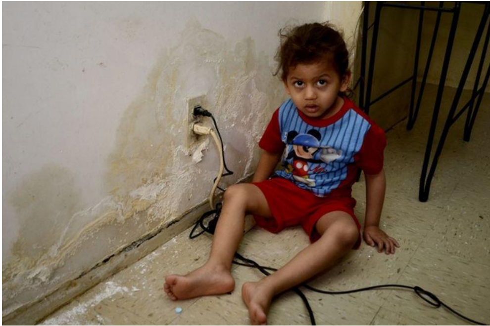
A child in a NYCHA apartment with mold on the wall. The New York City Housing Authority will come under federal judicial oversight over mold in apartments, enabling residents to go directly to a federal judge if the agency does not resolve the problem. (Richard Harbus for New York Daily News)
