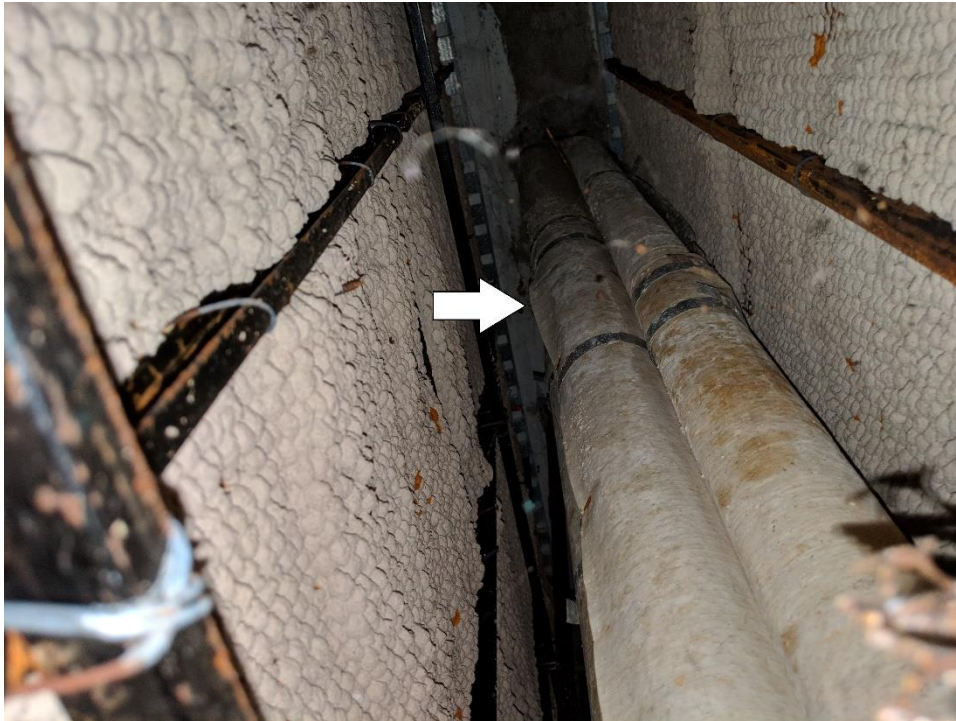
ACM- Pipe insulation (T.S.I)
