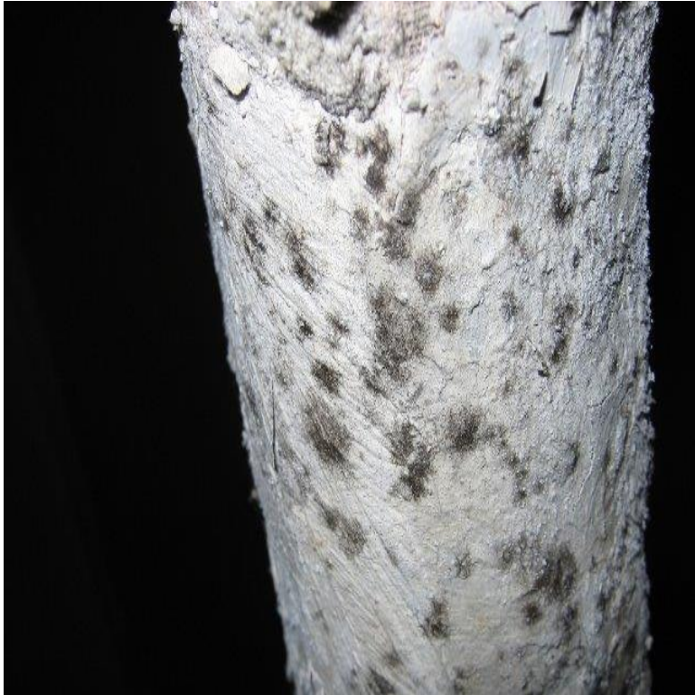
ACM- Pipe insulation (T.S.I)
