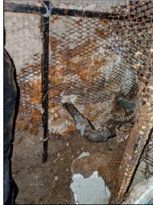
Missing insulation on cold water supply
