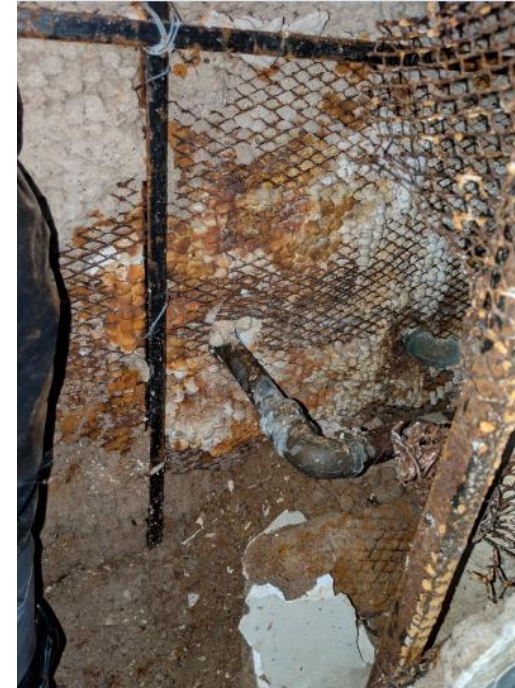
Missing insulation on cold water supply t
