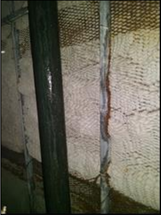
Missing insulation on cold water riser
