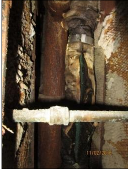
Damaged insulation on cold water riser
