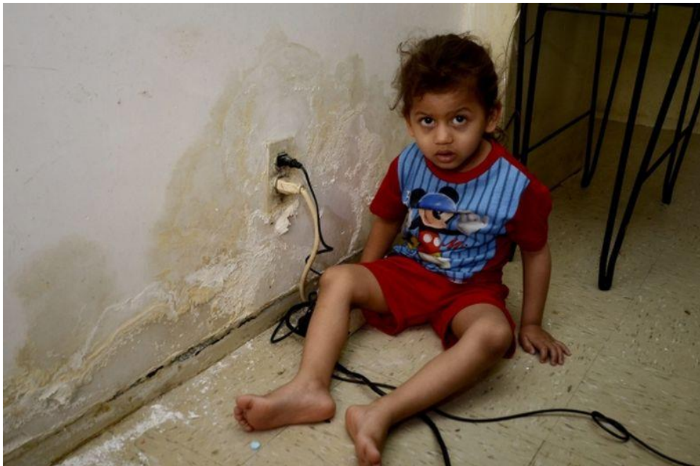
A child in a NYCHA apartment with mold on the wall. The New York City Housing Authority will come under federal judicial oversight over mold in apartments, enabling residents to go directly to a federal judge if the agency does not resolve the problem. (Richard Harbus for New York Daily News)
