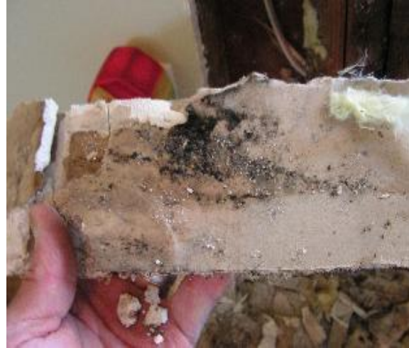
ACM- Spackle/Joint compound
