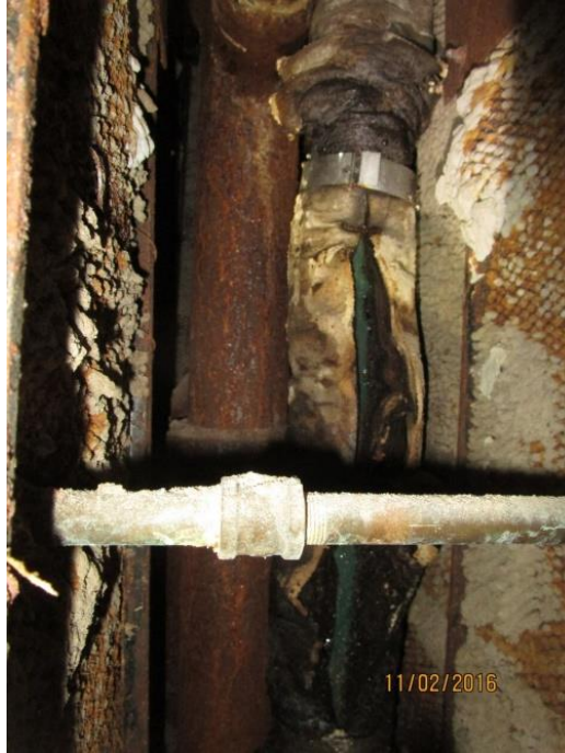
Damaged insulation on cold water riser
